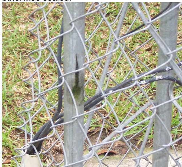
Rohn 25 - Split tower legs can be caused by improper water drainage and subsequent freezing. It's a sure-fire way of total failure.
