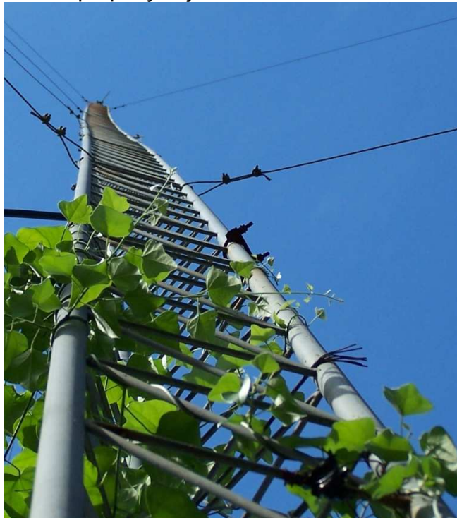
Tower bow can be caused by missing and improper guy wire tension. Notice the bow caused by imbalance number of guys on this tower photo.
